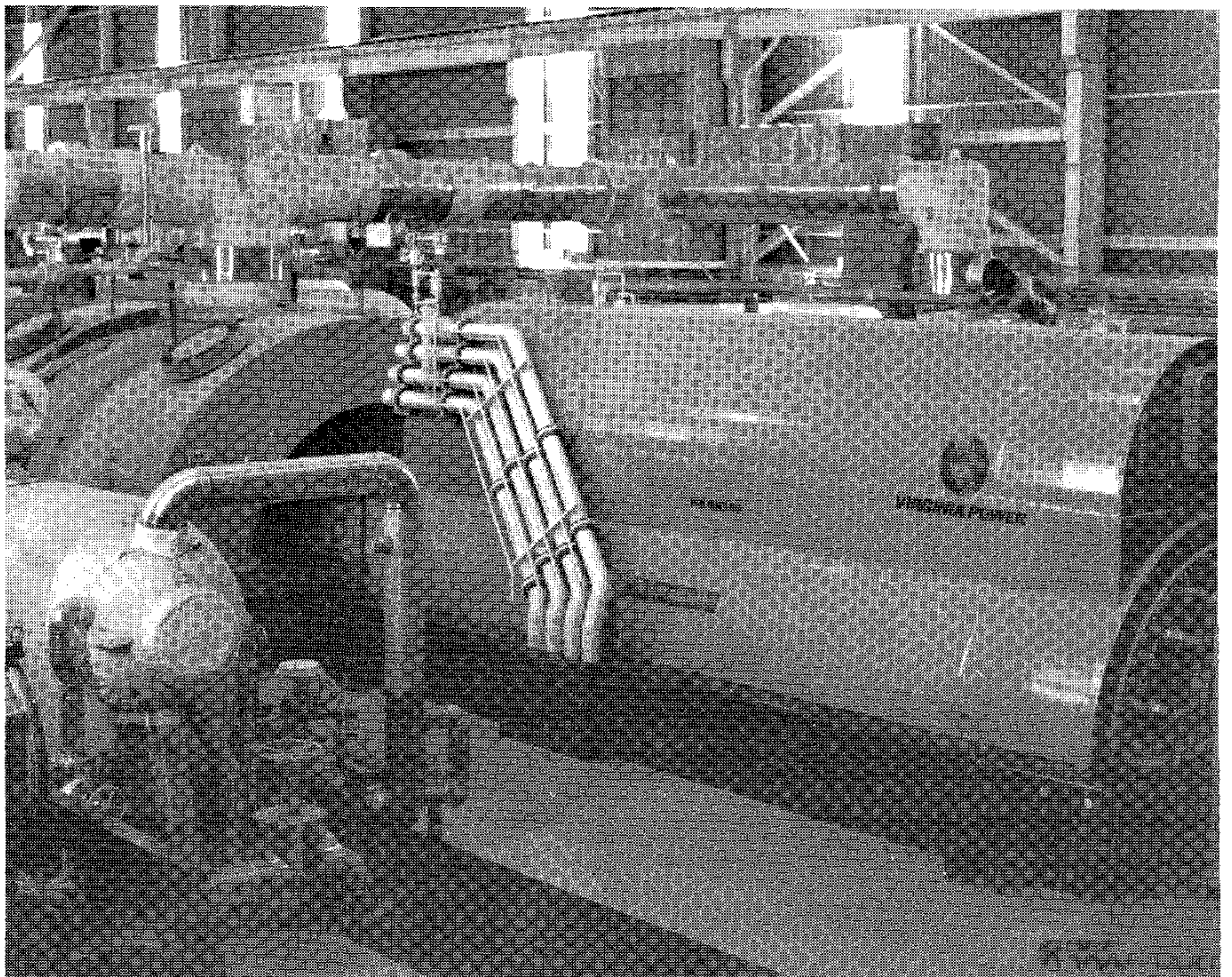
Fig. 19. The main turbine
