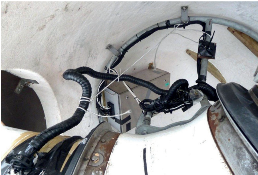
The data acquisition hardware was mounted in a single rack and secured in a waterproof box in the rotor housing. A slip ring was used for power transmission. Data was transmitted wirelessly to the PC in the tower, and synchronized using an IrigB time code
