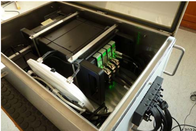
Fig. 7. LAN-XI modules installed in waterproof box
