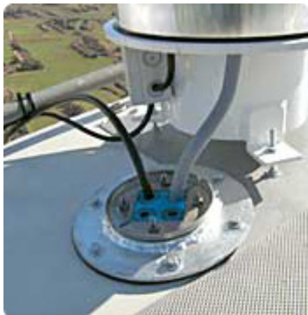
The sealing system on a wind turbine
